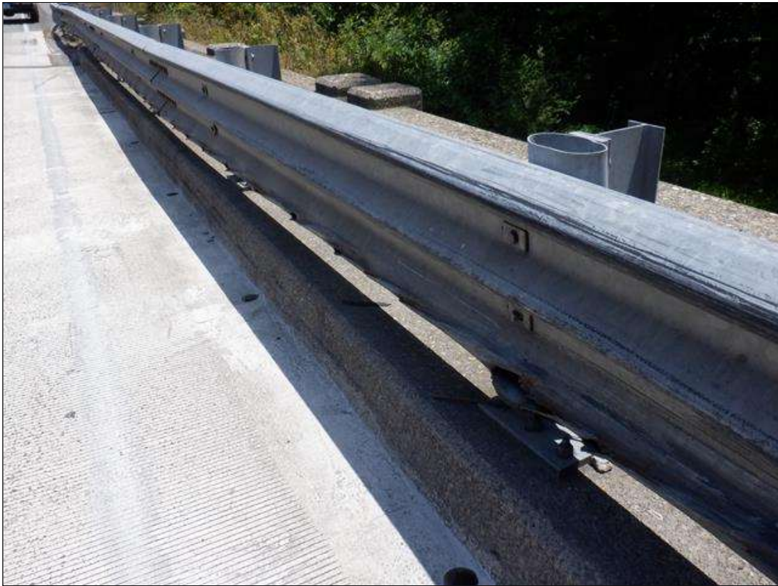
Span 8 Right Retrofit Bridge Rail: PAR, HEAVY IMPACT DAMAGE WITH UP TO 3 INCHES LONG X 1 INCH HIGH HOLES AND DENTS IN THE BOTTOM OF THE RAIL AND DEFLECTION UP TO 5 INCHES FOR FULL LENGTH
