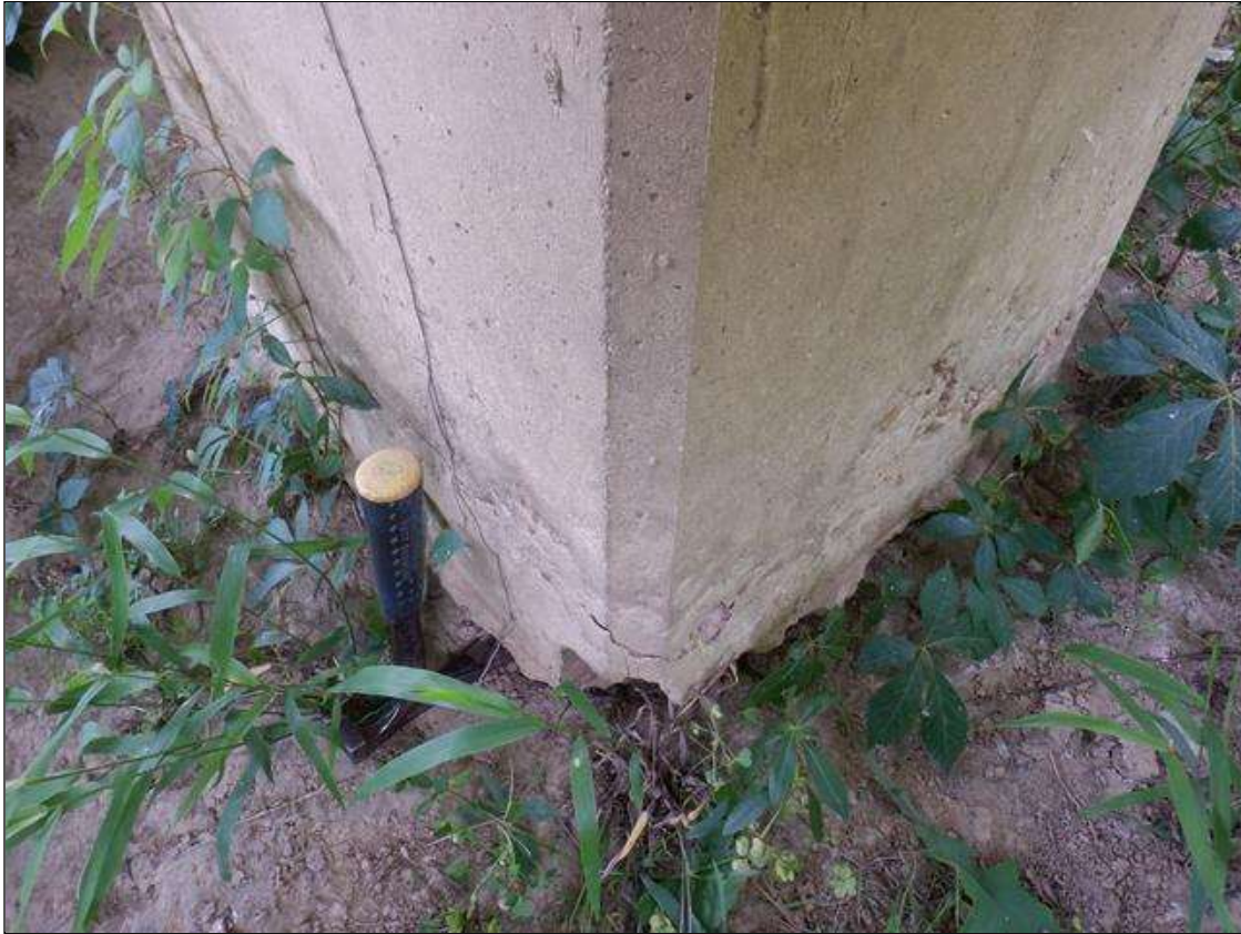
Bent 7 Pile 6: UP TO 3 INCHES HIGH OF THE STEEL PILE EXPOSED AT THE BOTTOM EXHIBITS HEAVY SURFACE CORROSION WITH NO MEASUREABLE SECTION LOSS IN THE FLANGES AND WEB. CONCRETE REPAIR AT BASE OF PILE COVERS STEEL PILE.
