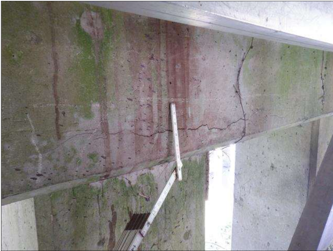
Bent 7 Cap 1: 3 FEET WIDE X 6 INCHES HIGH DELAMINATION WITH A 3 FEET LONG HORIZONTAL CRACK UP TO 1/16 INCH WIDE BOTTOM OF NORTH FACE, OVER PILE 3.
