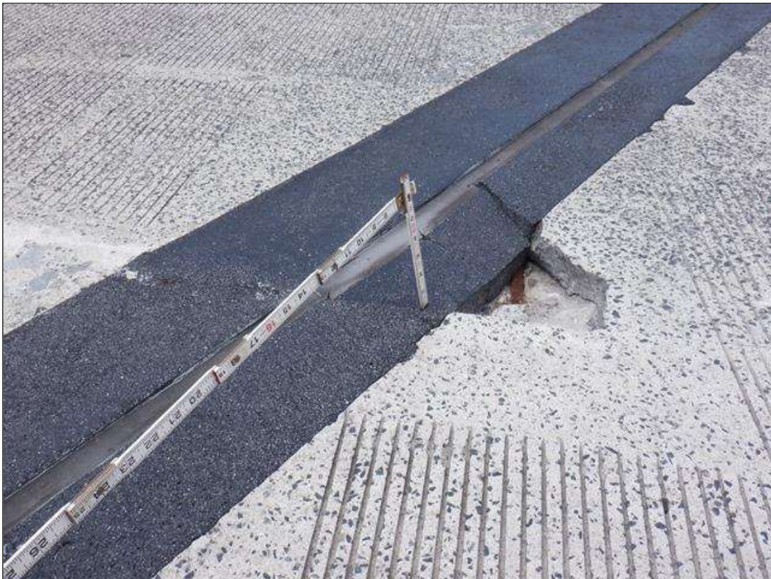
Span 6 Expansion Joint, Bent 5: ADJACENT TO DECK SPALL IN SPAN 6, 8 INCHES AREA OF HEADER DEPRESSED BY 1 INCH.
