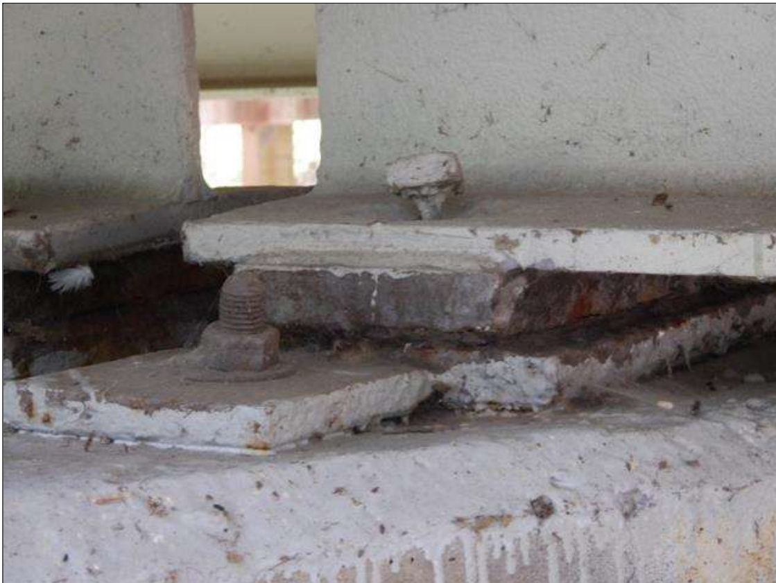
Span 8 Beam 4 - Near Bearing: SECTION LOSS EXISTS BENEATH THE PAINTED SURFACES IN BOTH MASONRY AND SOLE PLATES. UP TO 95 PERCENT SECTION REMAINING.
