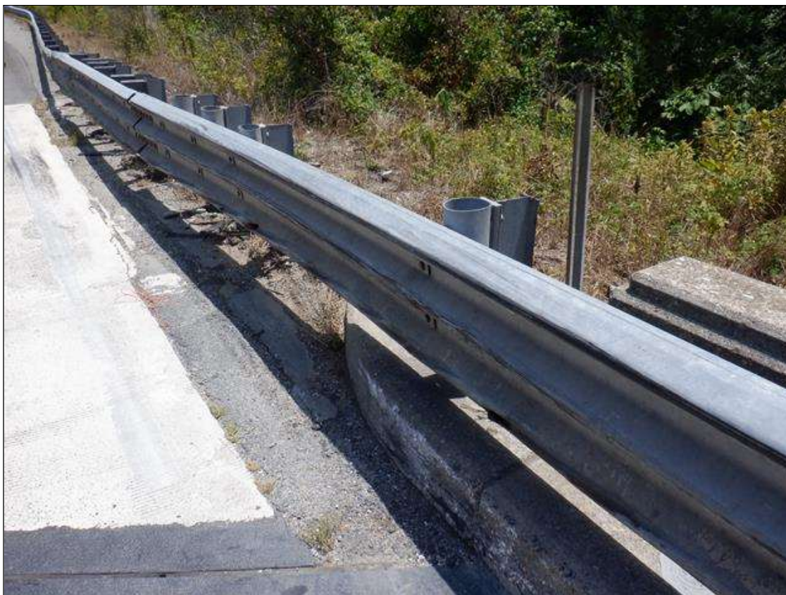
PAR. AT NORTHEAST CORNER IMPACT DAMAGE TO GUARDRAIL 50 FEET X UP TO 6 INCHES DEFLECTION.
