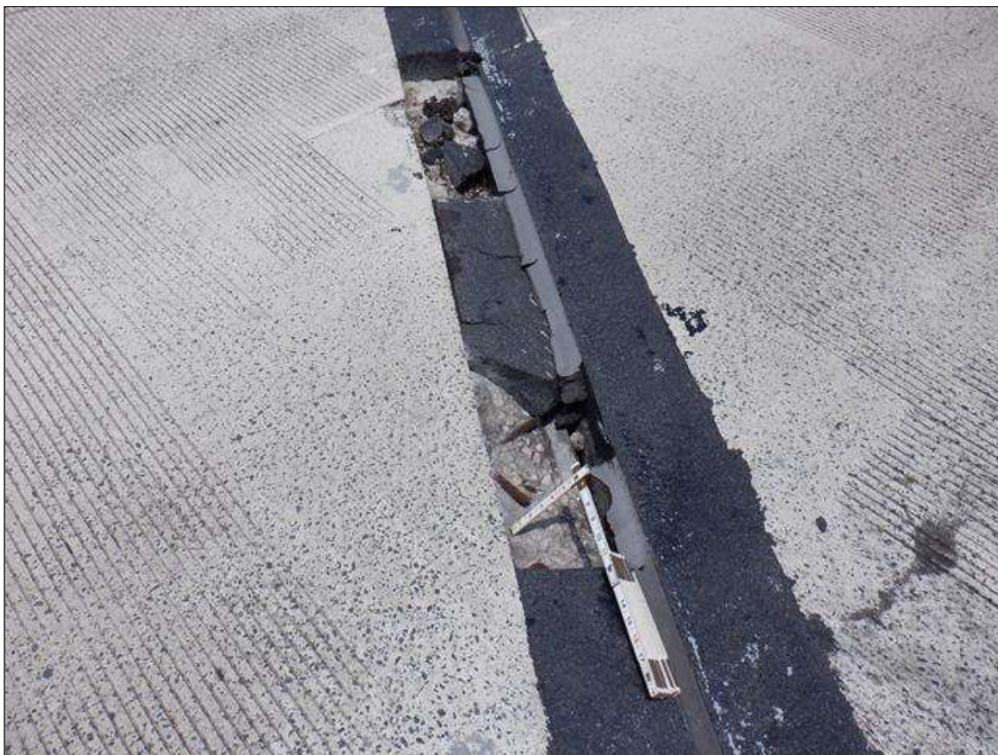
Span 7 Expansion Joint, Bent 6: PAR. IN RIGHT LANE 2 AREAS OF MISSING HEADER AND JOINT MATERIAL UP TO 2 FEET X 8 INCHES X FULL DEPTH.
