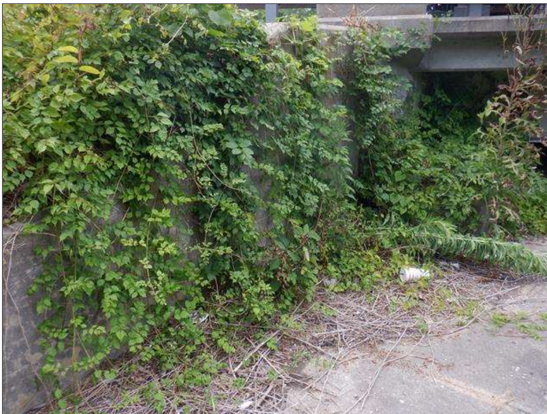
SOUTHEAST, SOUTHWEST, AND NORTHWEST WINGWALL HAVE VEGETATION GROWTH ALONG FULL LENGTH.
