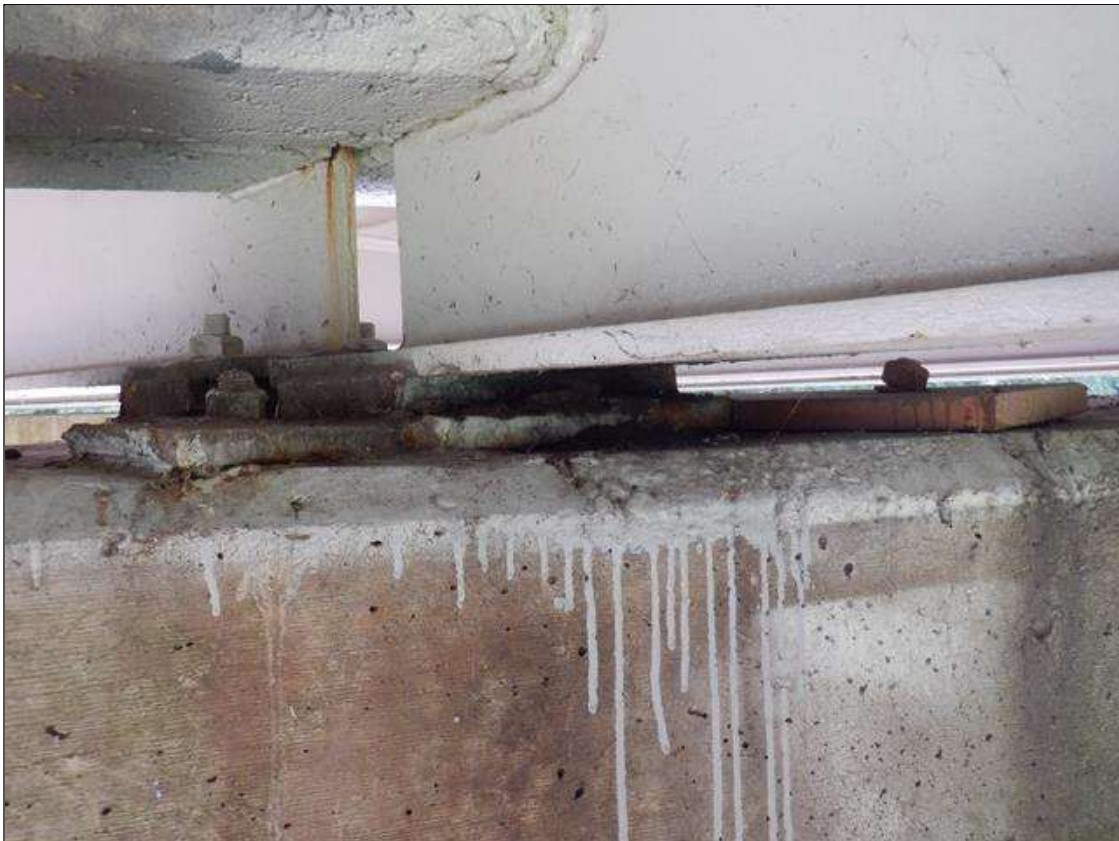
Span 4 Beam 2 - Far Bearing: WELDED REPAIR WITH ADDED ANCHOR BOLT.
