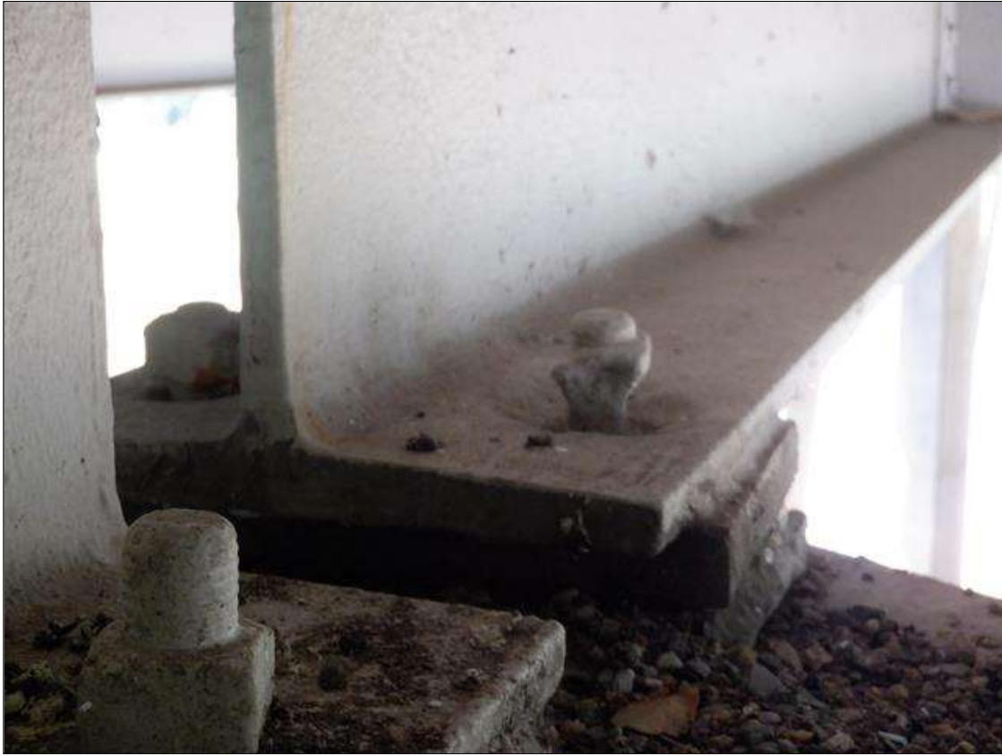
Span 6 Beam 3 - Far Bearing: LEFT ANCHOR BOLT HAS UP TO 80 PERCENT SECTION REMAINING AND ANCHOR BOLT NUT HAS UP TO 50 PERCENT SECTION REMAINING.
