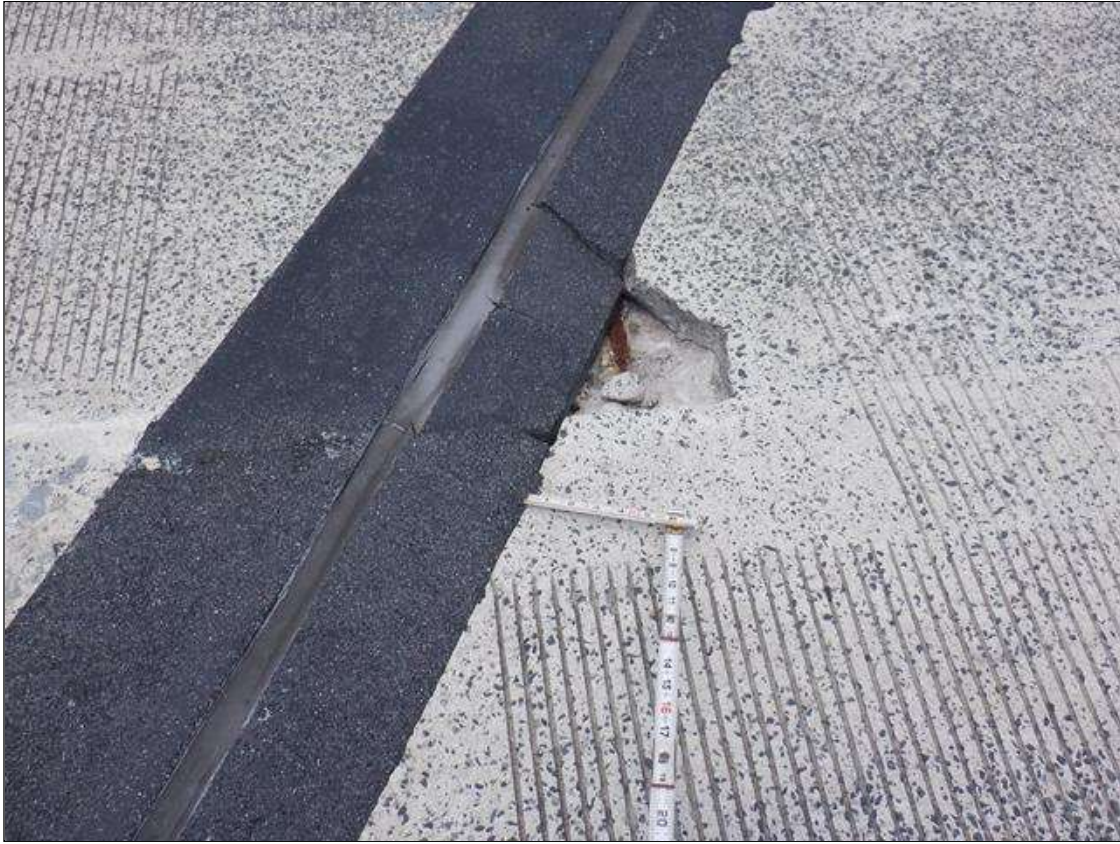
Span 6 Deck: PAR. AT CENTERLINE ADJACENT TO BENT 5, FULL DEPTH SPALL 8 INCHES DIAMETER WITH EXPOSED REBAR. NO SECTION LOSS.
