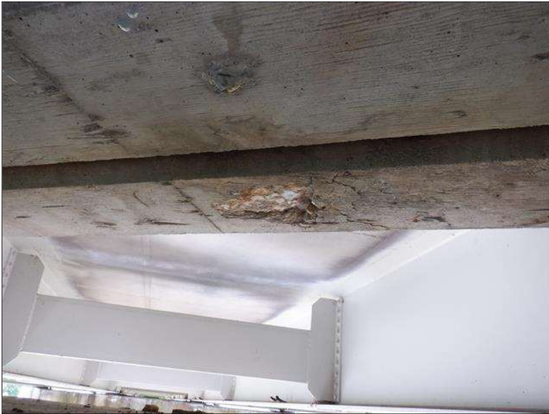
Span 5 Deck: 6 INCHES DIAMETER X 3/4 INCH DEEP SPALL IN INTERMEDIATE DIAPHRAGM IN BAY 2 ABOVE BENT 5.
