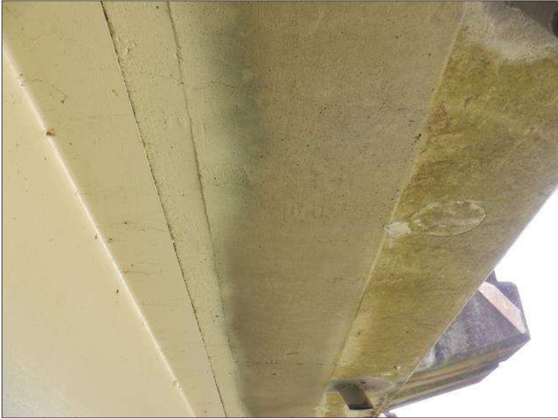
Span 1 Deck: SIX (6) UP TO 0.02 INCH WIDE TRANSVERSE CRACKS UNDER LEFT OVERHANG, SCATTERED.
