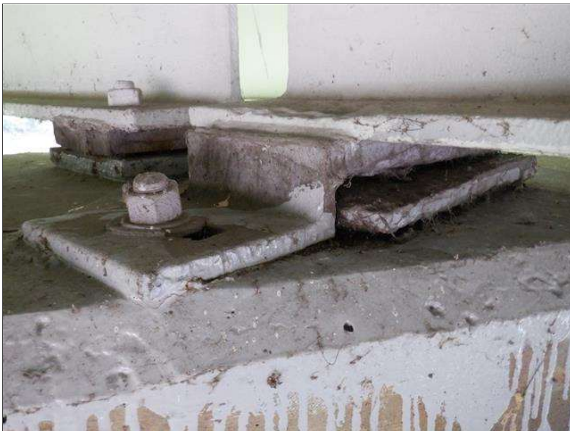
Span 1 Beam 3 - Far Bearing: WELDED REPAIR WITH ADDED ANCHOR BOLT.
