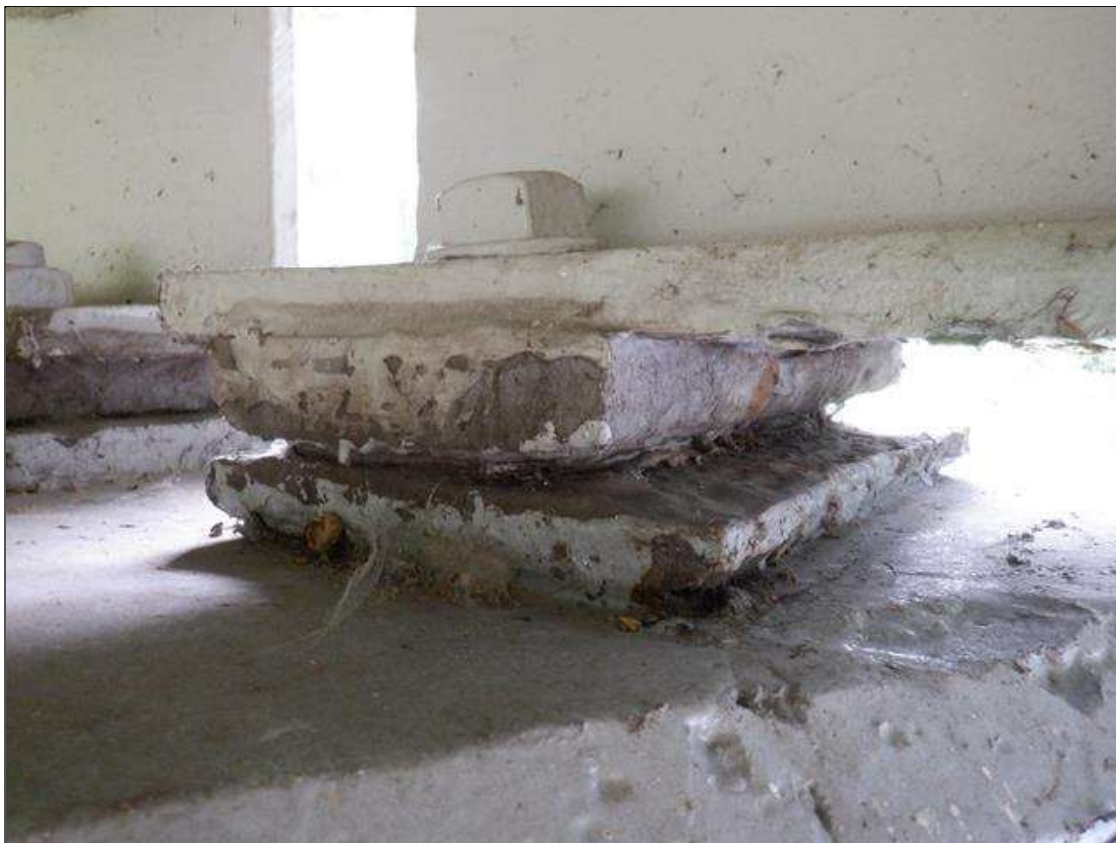
Span 1 Beam 4 - Far Bearing: SECTION LOSS EXISTS BENEATH THE PAINTED SURFACES IN BOTH MASONRY AND SOLE PLATES. UP TO 80 PERCENT SECTION REMAINING.
