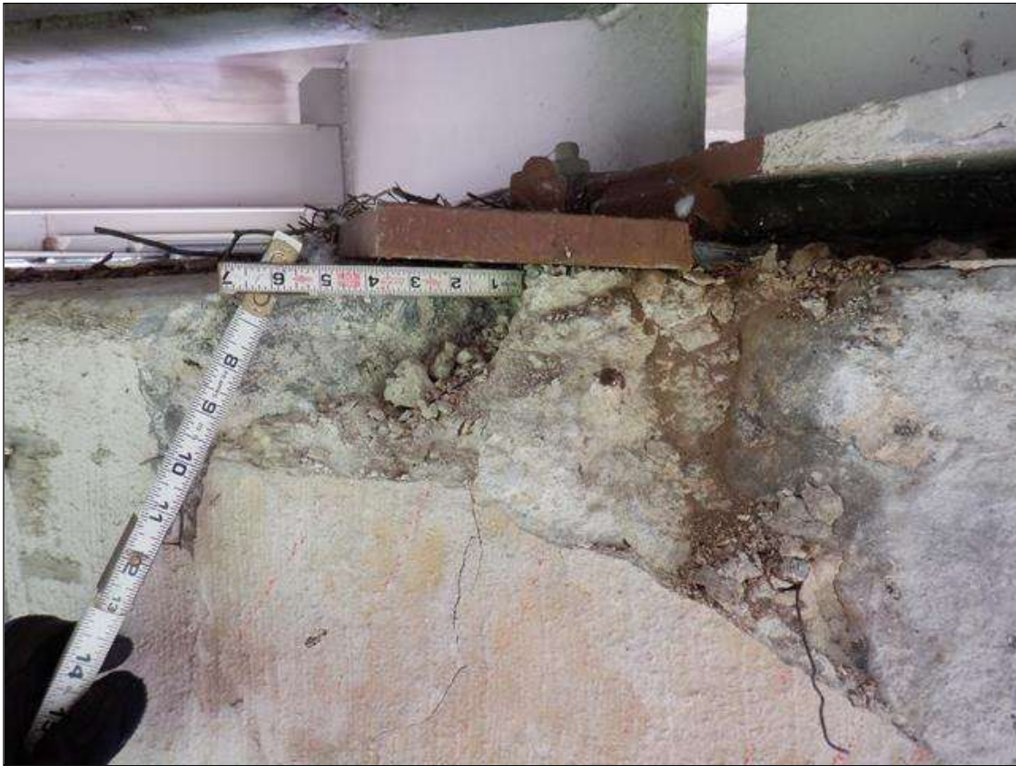
Span 4 Beam 3 - Far Bearing: PAR. ADDED BEARING HAS A LOSS OF BEARING AREA DUE TO SPALL ON CAP. AREA REPAIRED IS UNSOUND AND HAS 9 INCHES HIGH X 20 INCHES WIDE X 6 INCHES DEEP SPALLS.
