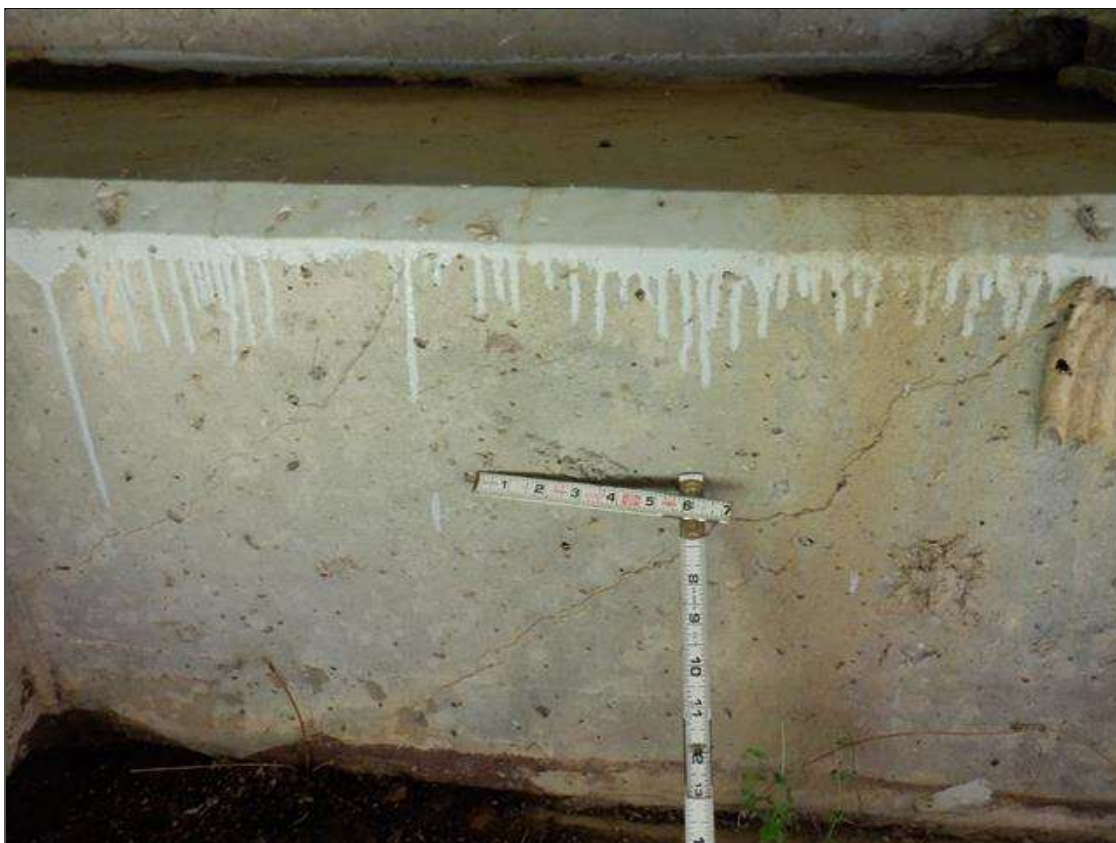
End Bent 1 Cap 1: TWO (2) 2 FEET LONG X 0.03 INCH WIDE DIAGONAL CRACKS IN FACE OF CAP BELOW BAY 2.
