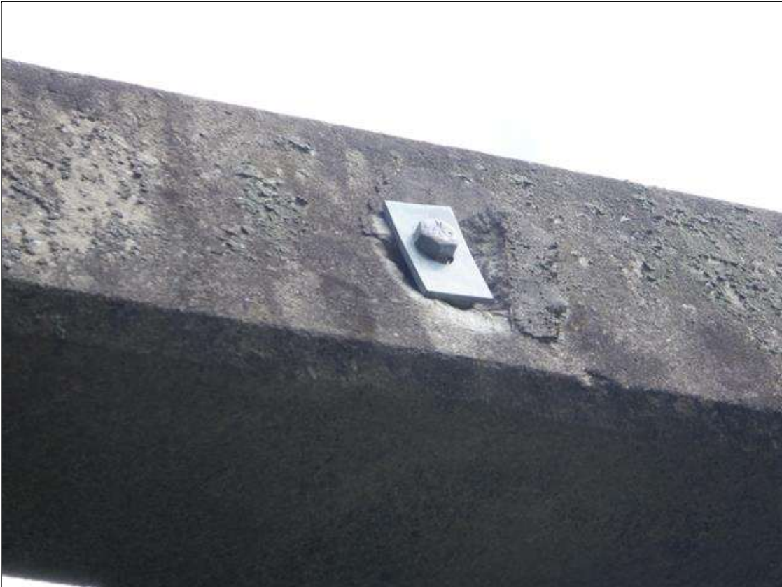
Span 1 Right Bridge Rail: UP TO 6 INCHES DIAMETER X 1.5 INCHES DEEP SPALL IN EXTERIOR FACE AT ANCHOR BOLT CONNECTION. TYPICAL AT SEVERAL CONNECTIONS.
