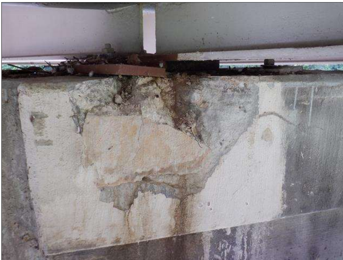
Bent 4 Cap 1: SOUTH FACE BELOW BEAM 3 UNSOUND PATCHED AREA WITH SPALLING 4 FEET X 18 INCHES, SPALLS 18 INCHES X 8 INCHES X 6 INCHES.
