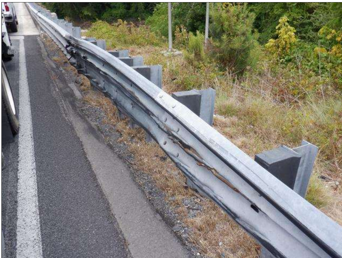
PAR. SOUTHEAST GUARDRAIL AT APPROACH HAS IMPACT DAMAGE 75 FEET LONG X UP TO 5 INCHES DEFLECTION.
