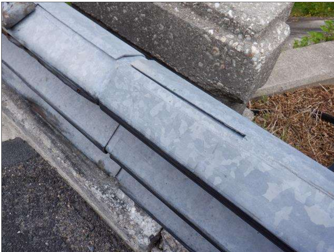
Span 1 Right Bridge Rail: AT END BENT 1, 2 SPALLS IN RAIL AND TOP OF CURB, 1 FOOT LONG X UP TO 4 INCHES X 4 INCHES
