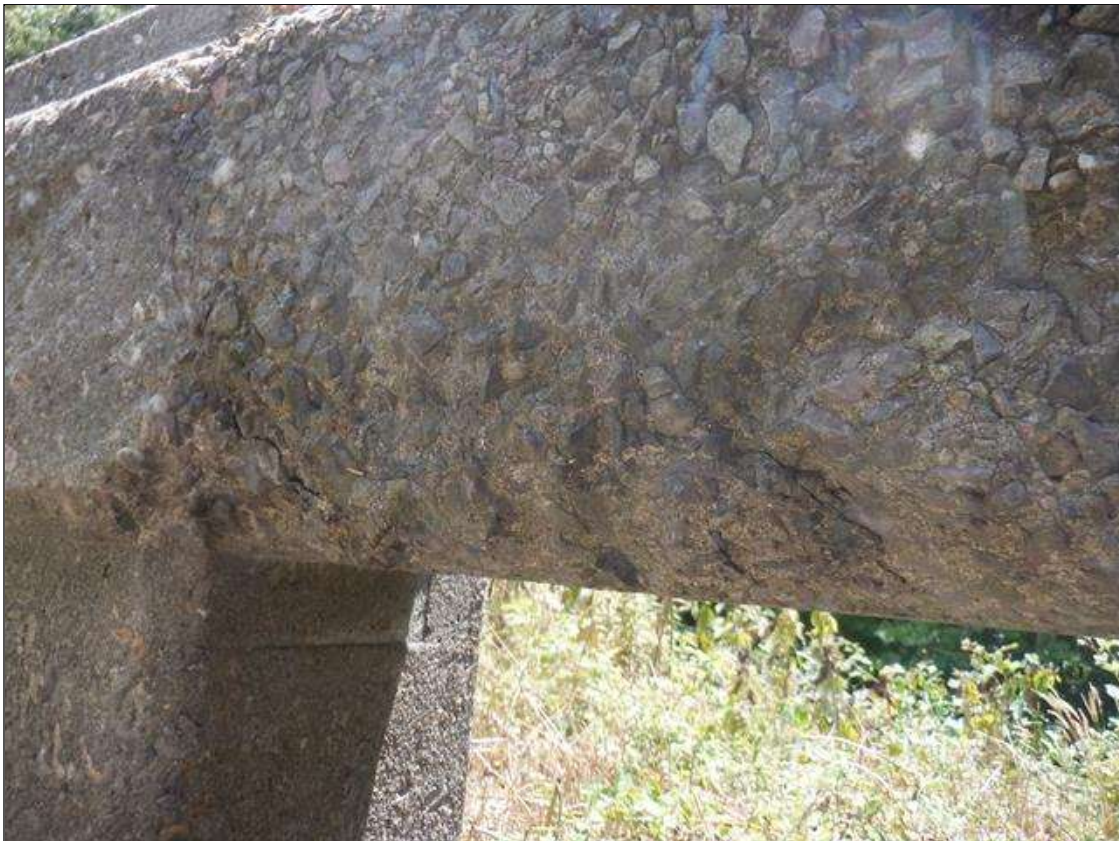
Span 8 Right Bridge Rail: 1 FOOT LONG X 4 INCHES WIDE X 1 INCH DEEP SPALL IN BOTTOM FACE AT END BENT 2
