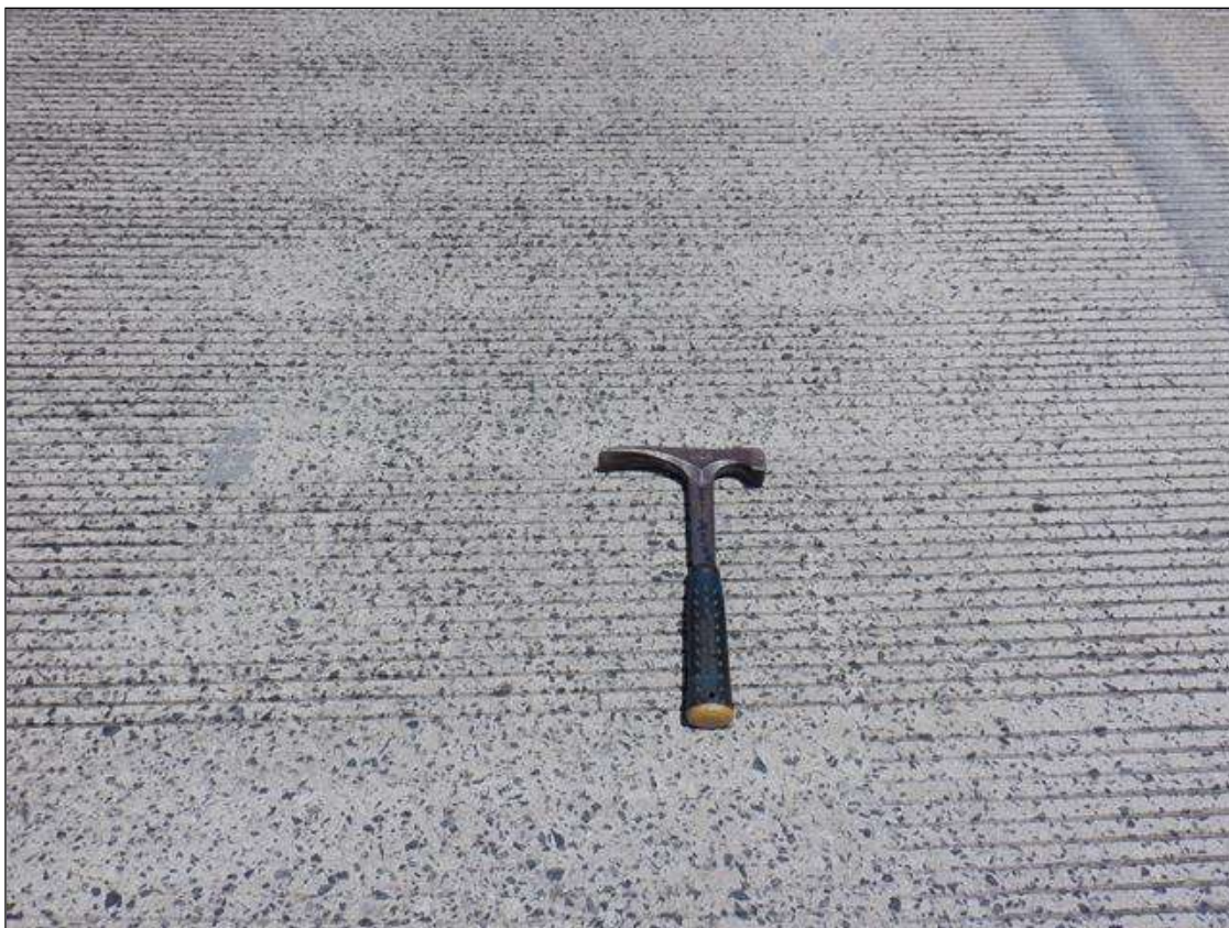
Span 8 Deck: MINOR ABRASION WITH EXPOSED AGGREGATE ALONG THE WHEEL PATHS FOR FULL LENGTH
