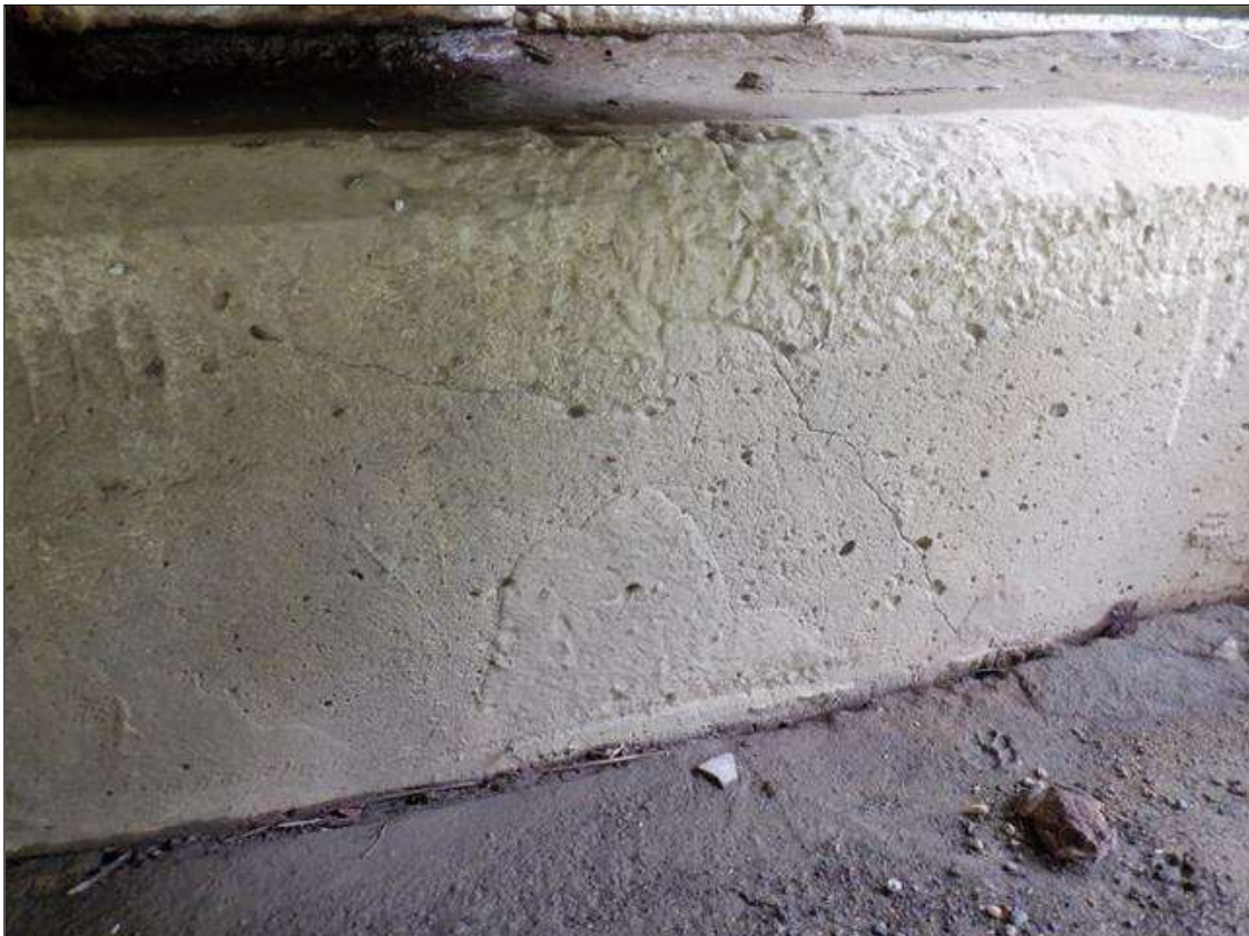
End Bent 2 Cap 1: 2 FEET HIGH X 1/16 INCH WIDE DIAGONAL CRACK UNDER BEAM 4.
