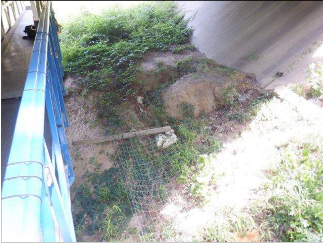
UNDER SPAN 8 AREA OF EROSION 20 FEET X 20 FEET X UP TO 3 FEET DEEP
