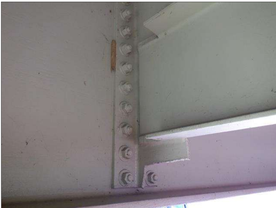
Span 1 Beam 4 : 2 INCHES HIGH OF INTERMEDIATE STIFFENER IS CUT OUT AT BOTTOM AT BOTH LOCATIONS. PAR IS NOT ISSUED AS IT APPEARS TO BE FROM PREVIOUS BRIDGE REPAIR.
