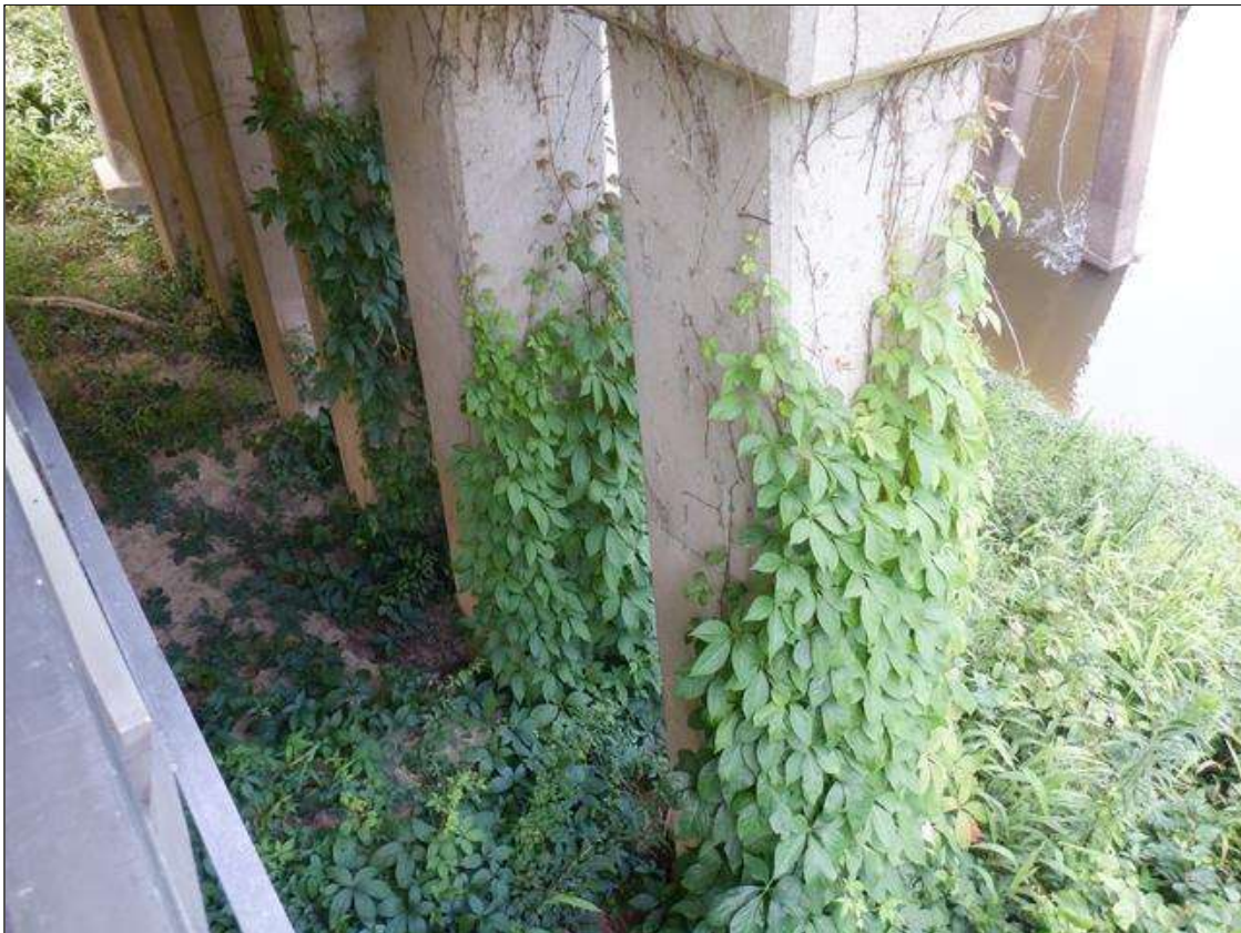
BENT 7 PILES 1 THROUGH 6 HAVE VEGETATION GROWTH UP TO FULL HEIGHT
