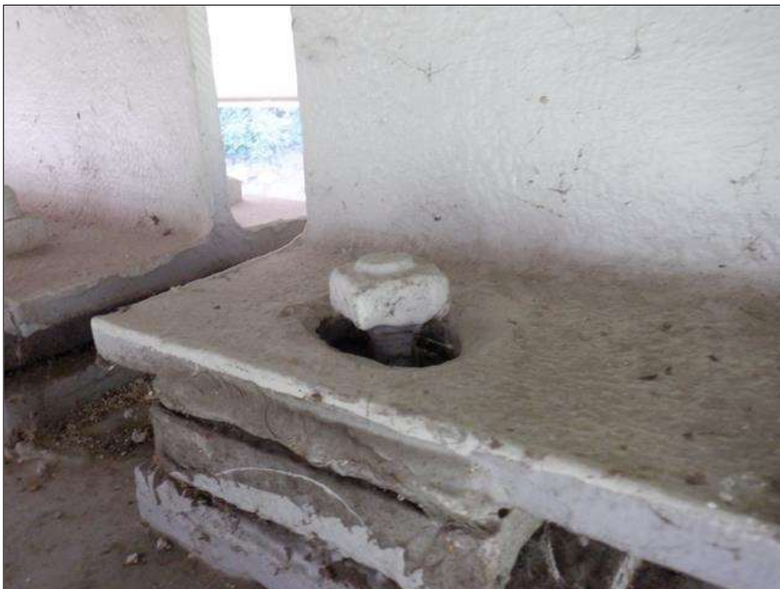
Span 3 Beam 3 - Far Bearing: PAR. ANCHOR BOLT NUT NOT CONNECTED COMPLETELY. SECTION LOSS WITH 70% OF BOLT REMAINING. HAS BEEN PAINTED.
