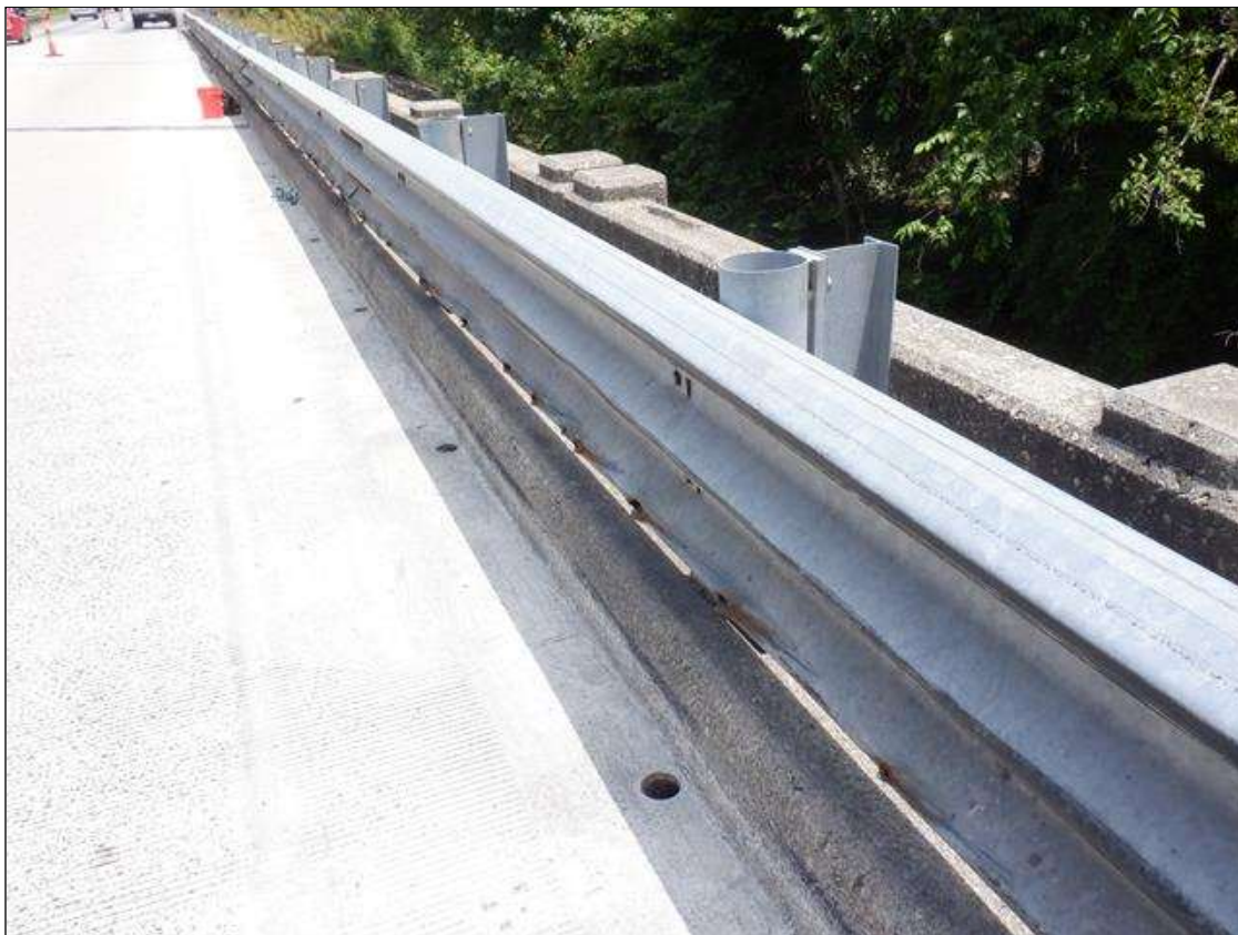
Span 6 Right Retrofit Bridge Rail: HEAVY IMPACT DAMAGE WITH UP TO 3 INCHES LONG X 1 INCH HIGH HOLES AND DENTS IN THE BOTTOM OF THE RAIL FOR FULL LENGTH
