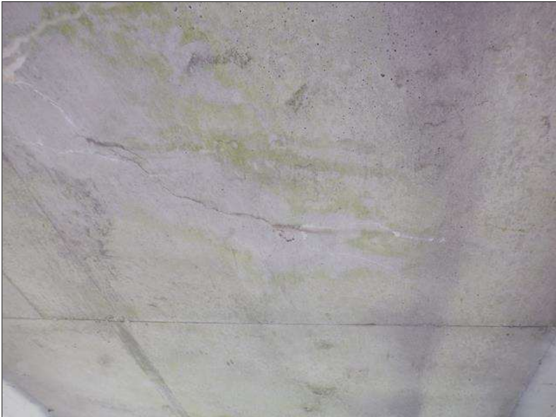
Span 1 Deck: UP TO 0.02 INCH WIDE TRANSVERSE CRACKS IN DECK UNDERSIDE IN BAY 1 BETWEEN INTERMEDIATE DIAPHRAGMS TYPICAL IN BAYS 2 AND 3.
