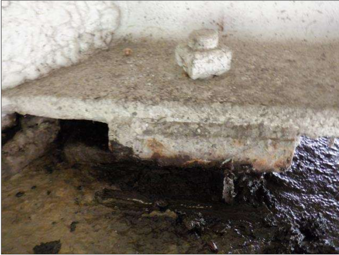
Span 8 Beam 4 - Far Bearing: UP TO 1/2 INCH MOVEMENT TOWARDS THE SOUTH LEFT HALF OF THE MASONRY PLATE.
