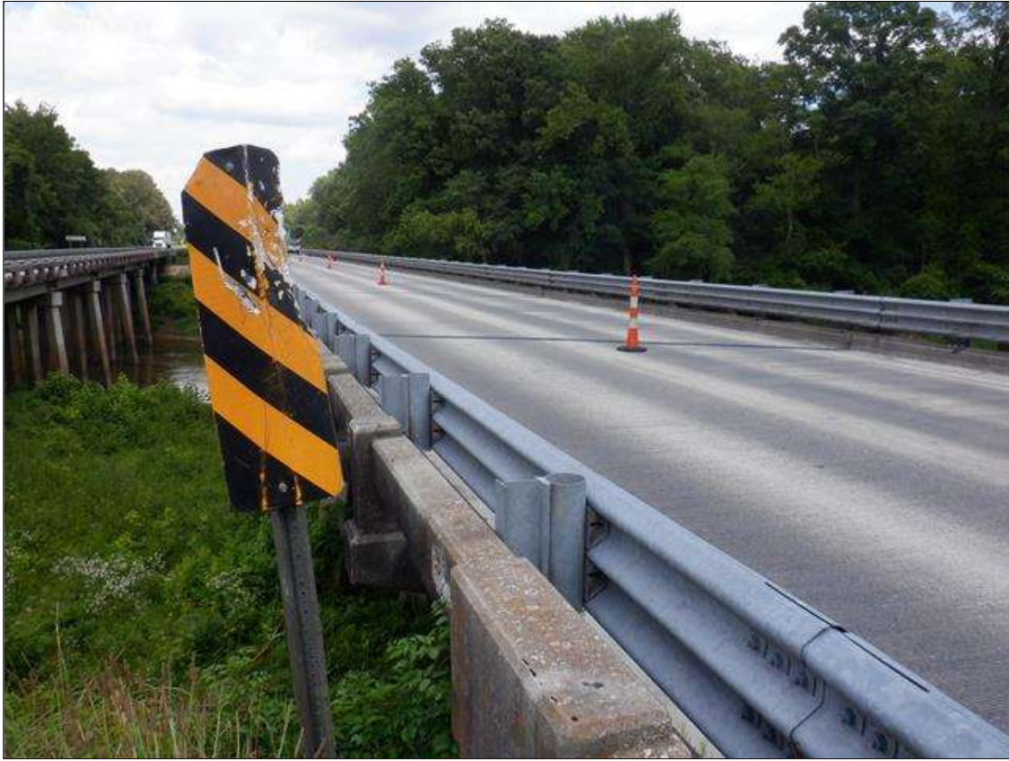
Span 1 Delineator SOUTHWEST: PAR. IMPACT DAMAGE TO SIGN WITH SCRAPING AND DISTORTIONS
