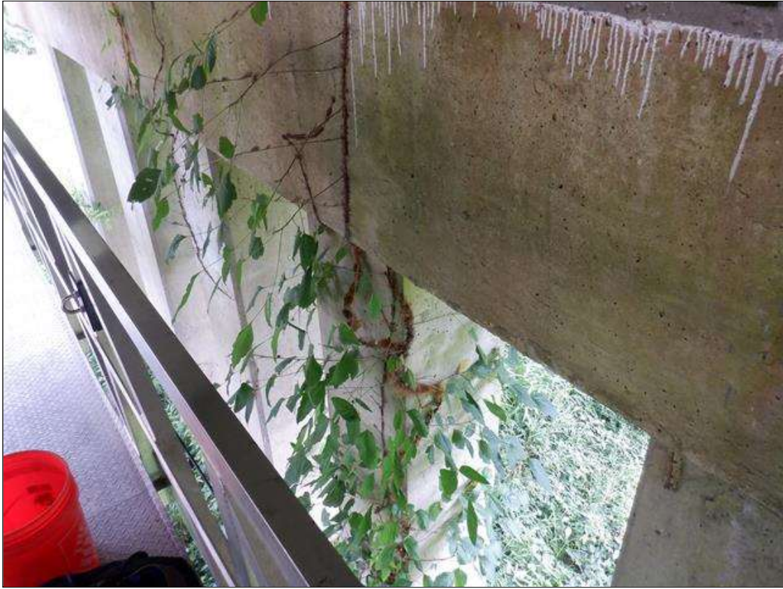
BENT 1 HAS VEGETATION GROWTH ON PILES AND CAP
